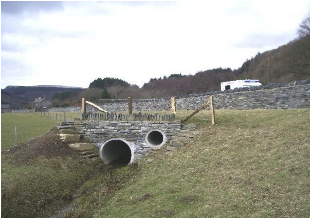
Otter dry pipe underpass adjacent to pipe culvert that may fill with water at time of flood. The wall alongside the road has overhanging coping stones to prevent otters from climbing over (Photo J. Jackson)
