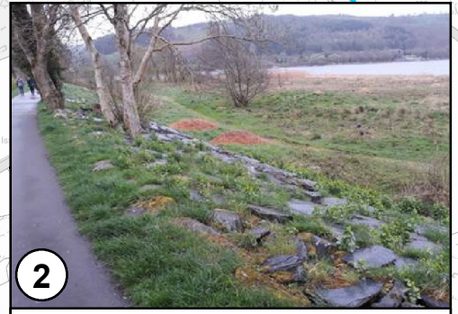
2 LAKE EMBANKMENT, LOOKING EAST ACROSS THE PROTECTED SITE; EVIDENCE OF RECENT WILLOW SCRUB CLEARANCE
