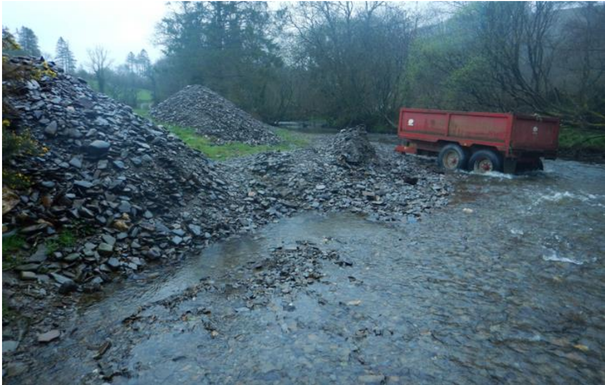
Figure 17 Trailer in a river carrying out illegal gravel removal. This is an example of unconsented river modifications (the example shown has occurred since 2017) (Source: NRW).
