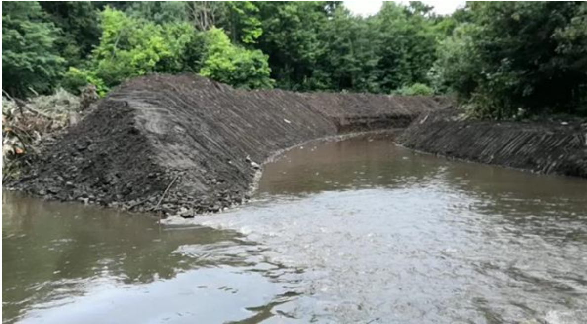
Figure 19 Reprofiling, dredging and levee creation, destruction of riparian corridor and in-channel features, severely degrading fish habitat and causing extensive siltation. This is an example of unconsented river modifications (the example shown occurred in 2020) (Source: NRW).
