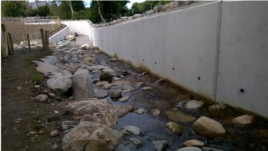
Figure 20 Example of channel engineering as a result of a local authority flood alleviation scheme constructed in 2016 (Source: NRW).
