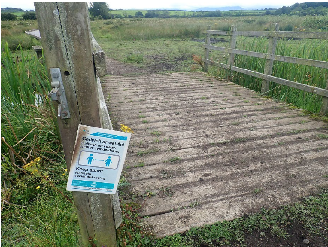
Timber bridge used to enable access by stock and pedestrians, Cors Bodeilio NNR, Anglesey. Photo: P.S. Jones
