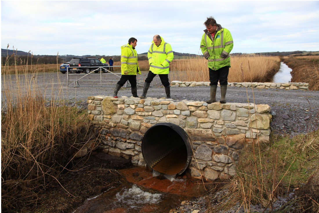
Stone and fill bridge with culvert over a deep boundary drain at Matharn Uchaf, Penllyn. The image shows Photo: P.S. Jones/Anglesey & Llyn Fens LIFE Project.
