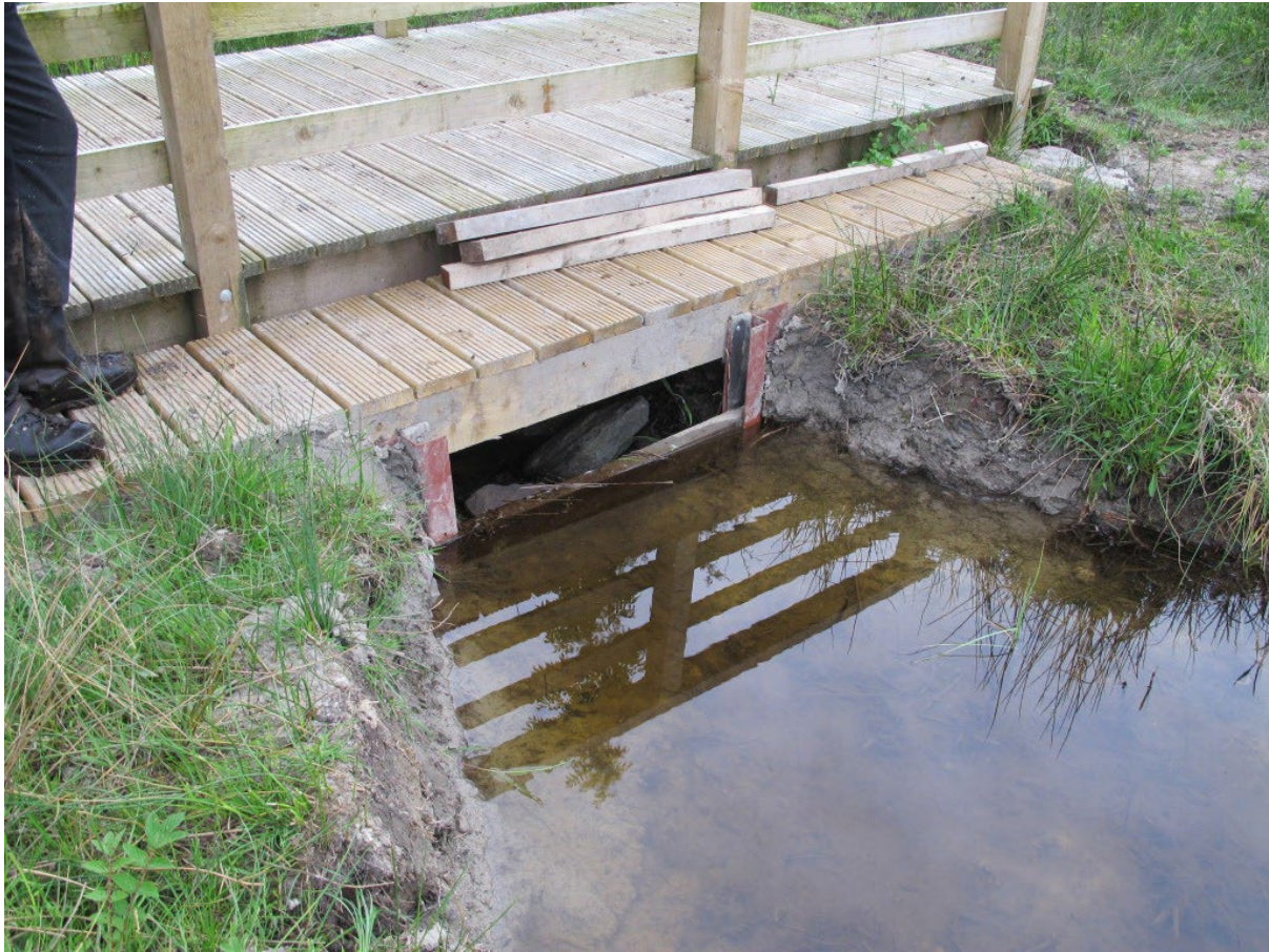
Adjustable weir installed together with a stock bridge and pedestrian bridge for access to enable adjustment or measurement. Drop boards can be added or removed to achieve target water levels. Cors y Farl SSSI, Anglesey. Photo: P.S. Jones/Anglesey & Llyn Fens LIFE Project.
