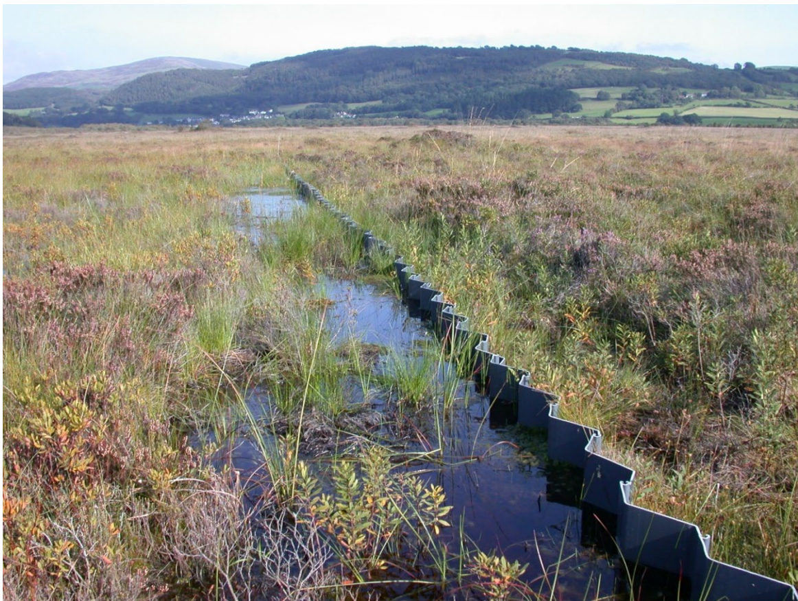
Plastic piling raising water levels in an old peat cutting. Cors Fochno, Ceredigion. Photo: P.S. Jones.
