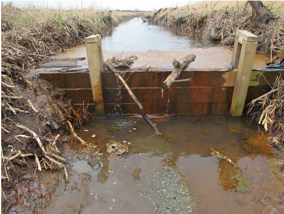
Simple timber sluice built in-situ to increase water levels in an over-deepened ditch, Cors Hirdre SSSI (Penllyn). Photo: P.S. Jones/Anglesey & Llyn Fens LIFE Project.
